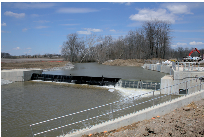
Inflatable Dam I bladder and gate slightly down
