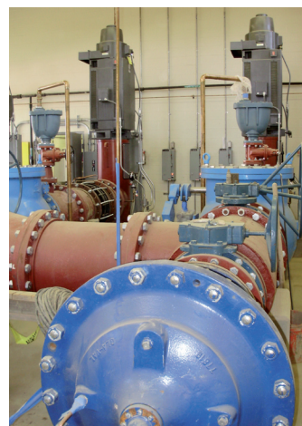
Inside the pump station, two vertical turbine pumps across piping and valves
