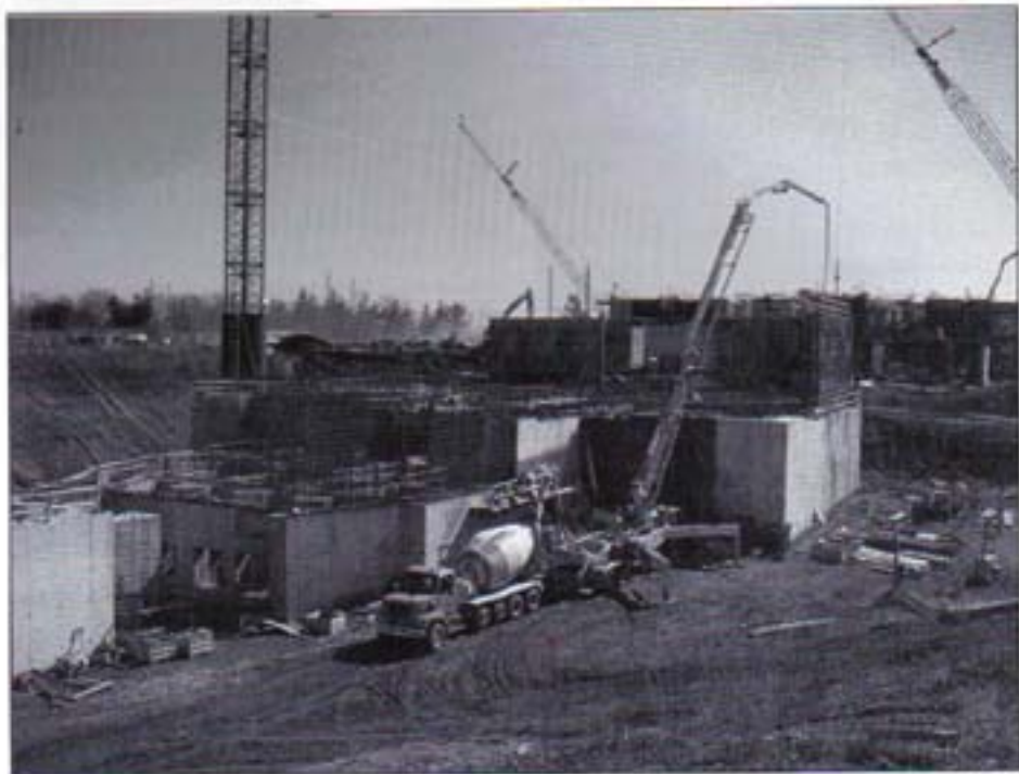
More than 50,000 yd 3 of concrete will be used to complete this expansion of the Southerly Wastewater Treatment Plant for Columbus, OH.
